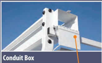
Conduit Box w/ Diamond Plate
